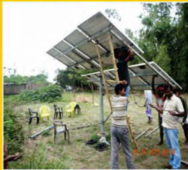
Locals setting up solar panels with the help of technicians in Kalikapur village
