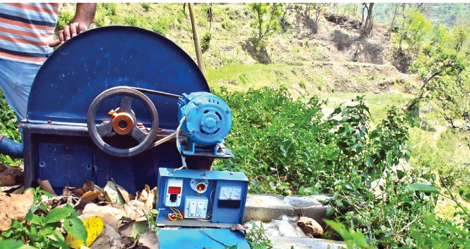
Tipli just recently installed micro hydel station that generates electricity for its farm to prevent crops from animal attacks.
